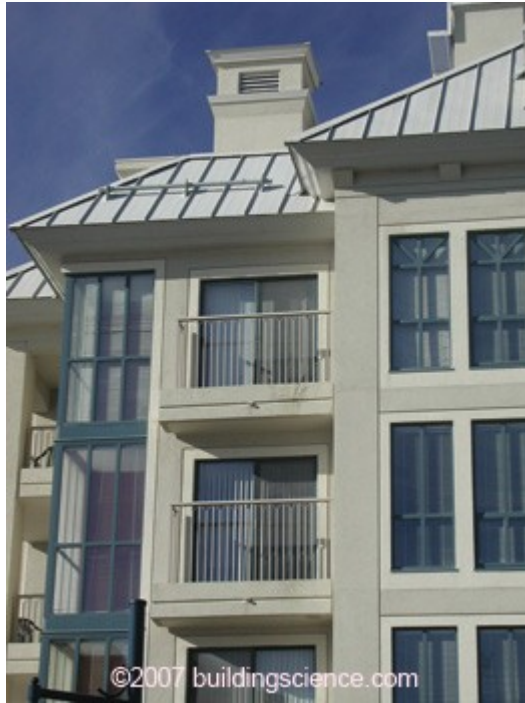
Photograph 1: Architectural details such as overhangs, balconies, and railing connections contribute to the amount of rain deposited in or on a wall
