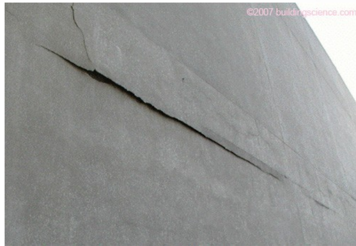
Photograph 3: Frame shrinkage at the rim joist of this wood-framed building caused the stucco to buckle
