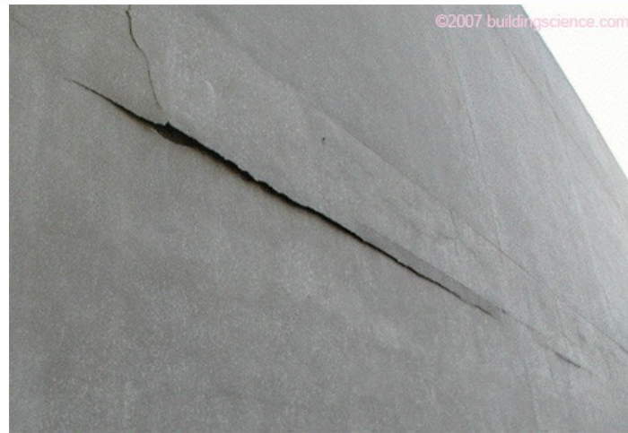
Photograph 3: Frame shrinkage at the rim joist of this wood-framed building caused the stucco to buckle
