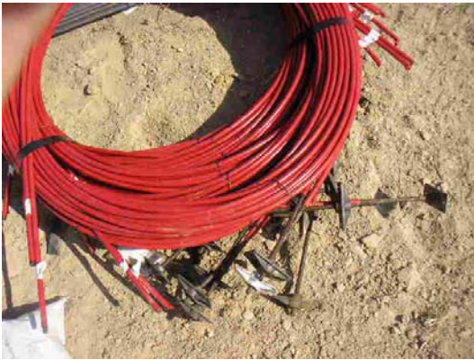
this is a bundle of post-tensioning cables as they are delivered to the site
