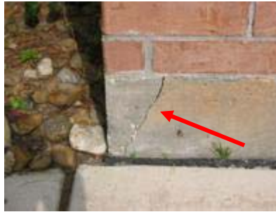
corner or wedge crack
