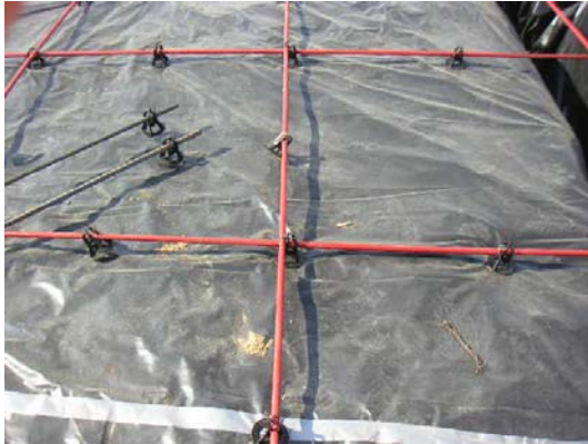
this is a close-up of the post-tensioned cables after installation – notice the conventional reinforcing steel at the left side; it is not unusual to mix post-tensioned and conventional reinforcing
