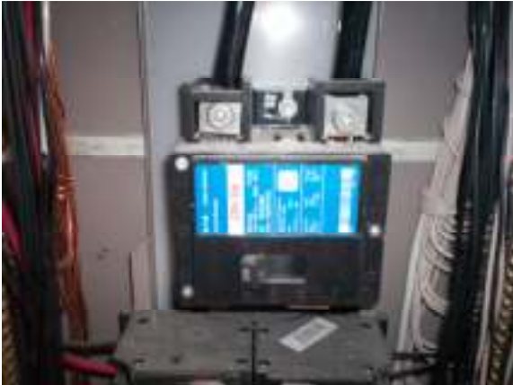
Main Power/Cable Entrance Underground. 200 Amp Main Panel Breaker box with main disconnect is located in the garage interior.
