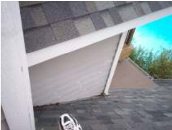
As seen at the rear slope on the roof, the siding is too close to the shingles and has caused a damming effect. Recommend the siding be raised up to 2" and the debris be removed. You will need to monitor this area and clean out any debris that accumulates and slows the water runoff.
