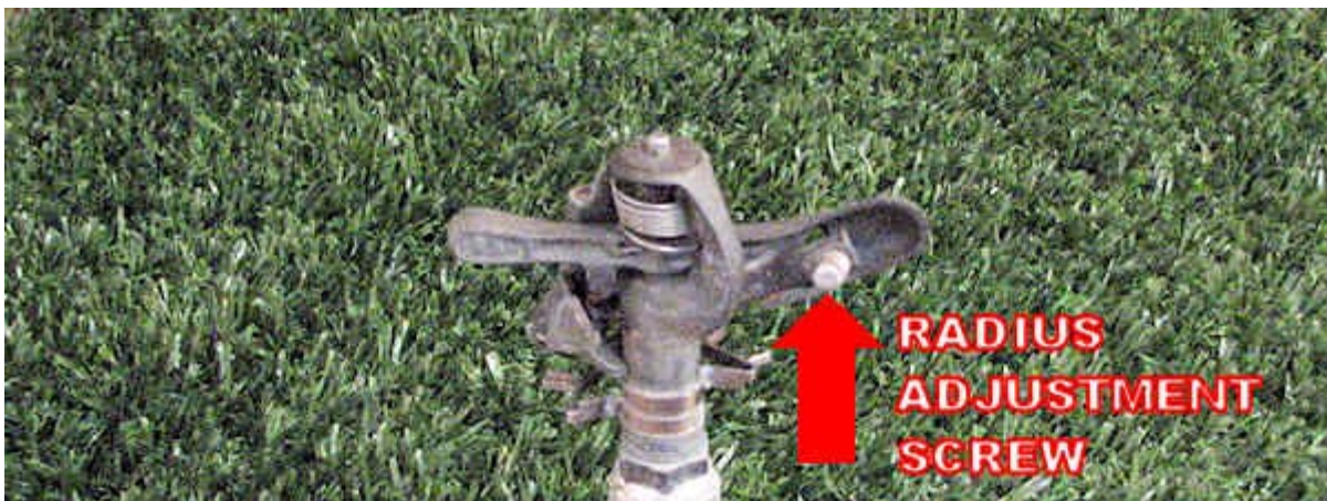
Impact Driven Rotor (mounted on pipe above ground)
