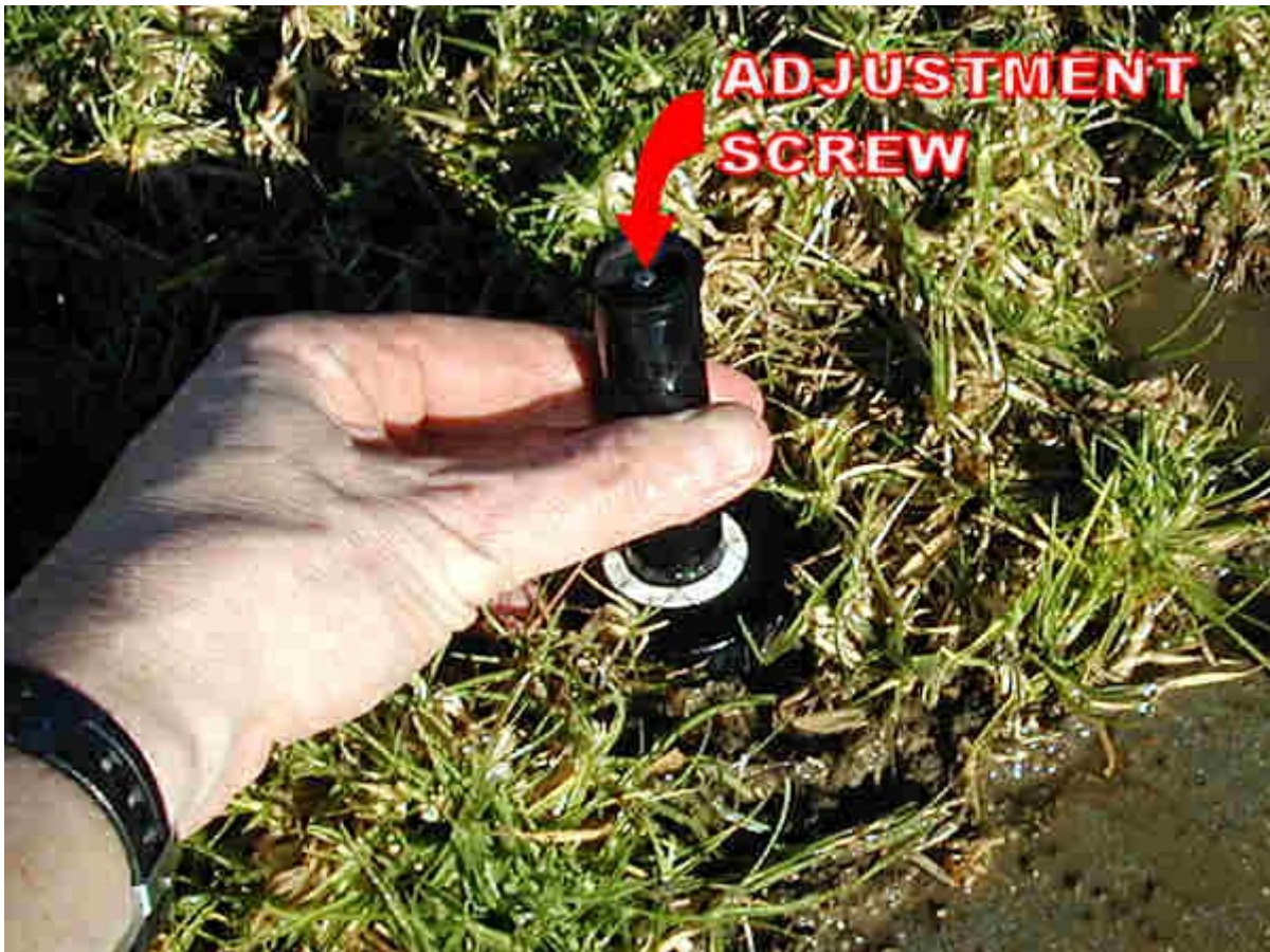
Adjustment Screw on a Spray-Type Sprinkler
